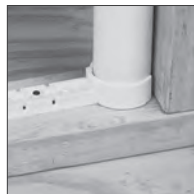
Glue to DWV pipe to support vertical runs.
