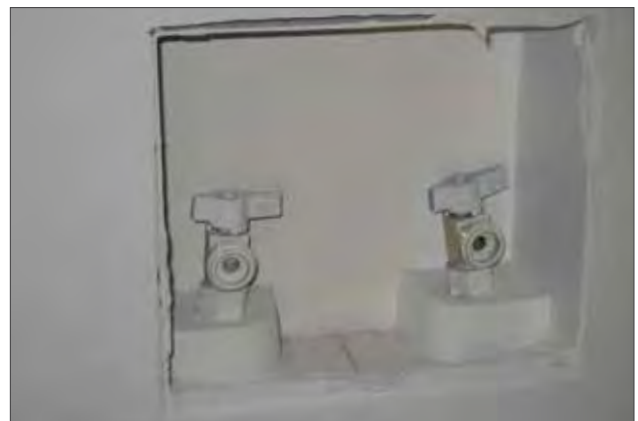
Unprotected Opening. Open boxes are susceptible to drywall mud, paint, dirt and debris or require added time and material to protect them.
