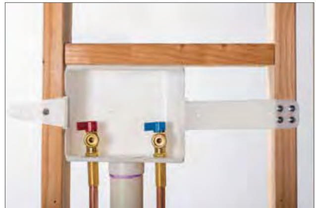
Inferior Bracketing. Contractors are forced to add their own wood braces to supplement flimsy styrene brackets.
